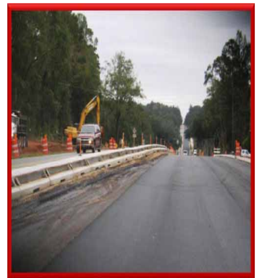
US 90 (Mahan Dr.) asphalt placement. Photo is looking eastbound in front of the Stormwater pond.
