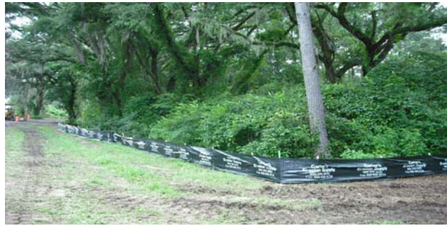
Silt Fence Protects the Trees from Erosion Control Damage.
